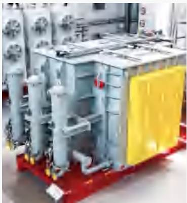
Transformer for Electric Arc Furnace at Zhanjiang Steel
