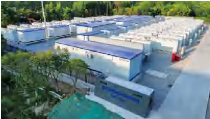
The first energy storage project within the Baosteel industrial site
